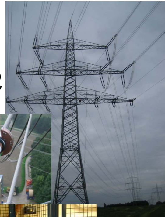
Test of communication range on 380kV power line
